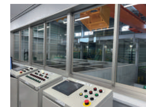
An internal view of the soon-to-become-operational smart plant
